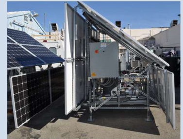
VariSun Solar Vapor Extraction Systems
