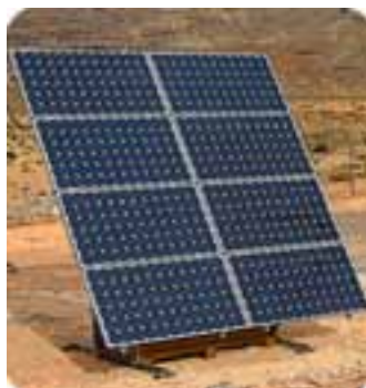
Stand Alone Solar Leachate Pumping System
