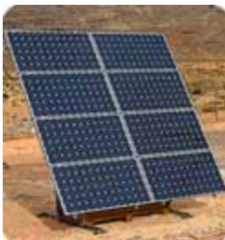
Stand Alone Solar Leachate Pumping System
